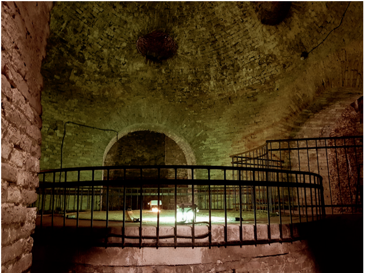
Fig. 56. Great Well in the Belgrade Fortress – working platform over the dry shaft in the protective entrance structure (PE Belgrade Fortress)
