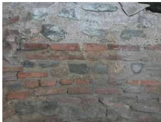
Fig. 3 Bricks in wall facing of Viminacium thermae. Photo-documentation of Institute of Archaeology Belgrade
