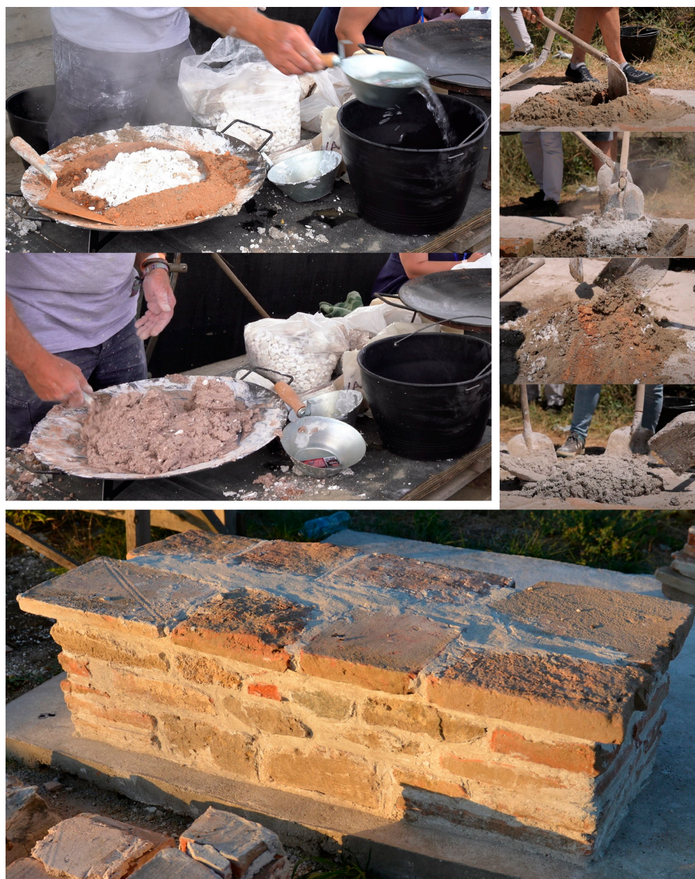
Figure 13. Hot mixing during the MoDeCo2000 workshop. Creating a demonstration mixture ( top left ) and the mixtures for a wall structure using lime mortars, with natural brick as admixture with a photo of the wall 11 days after the building ( top right , and bottom ). Photo documentation of the MoDeCo2000 project.
