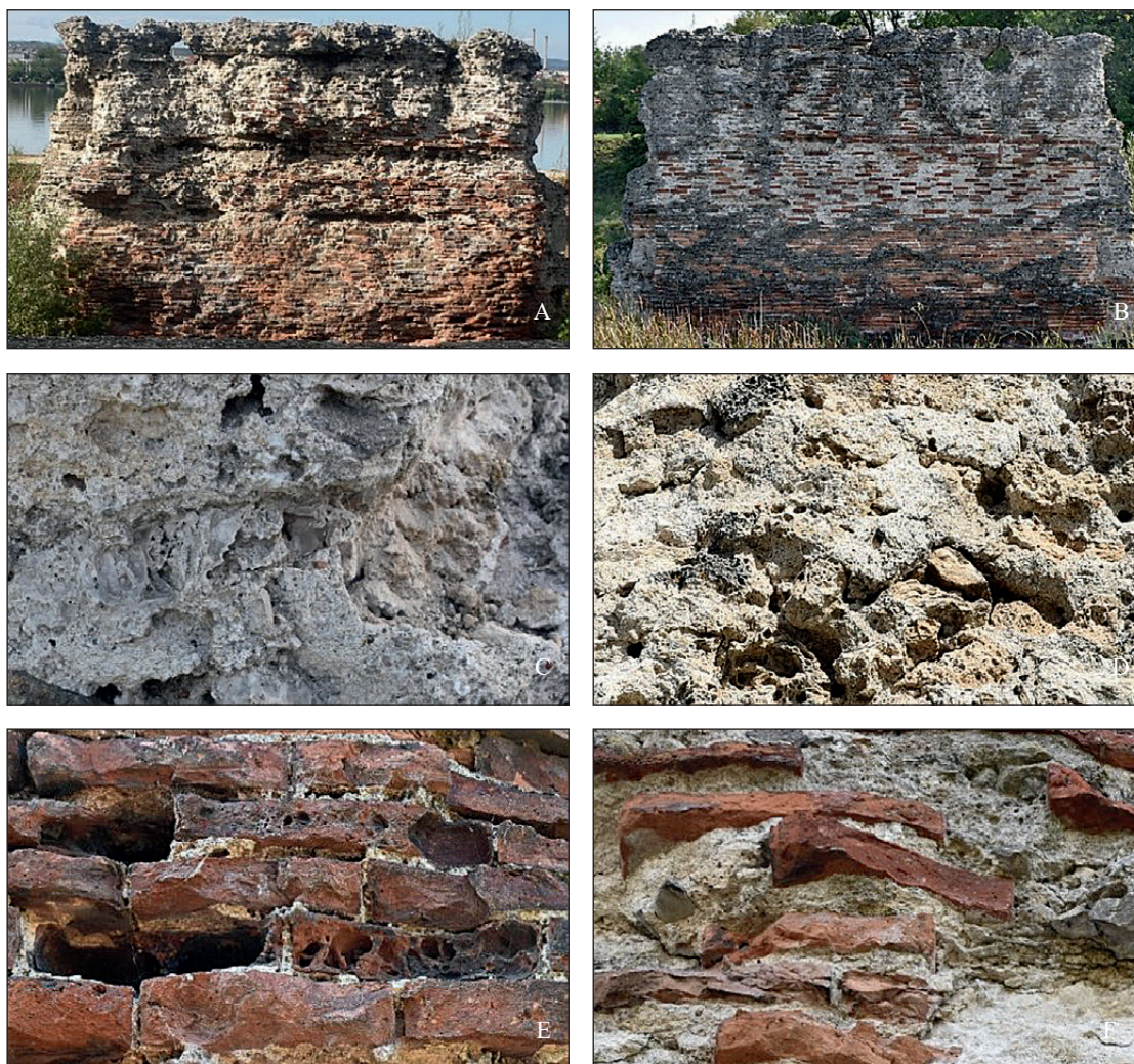
Fig. 5. Deterioration of the pillar – southern side in 2020 (A), and northern side in 2022 (B); stone and mortar deterioration in 2020 (C, D); brick and mortar deterioration in 2021 (E), and in 2022 (F) (Archive of the MoDeCo2000 project)
