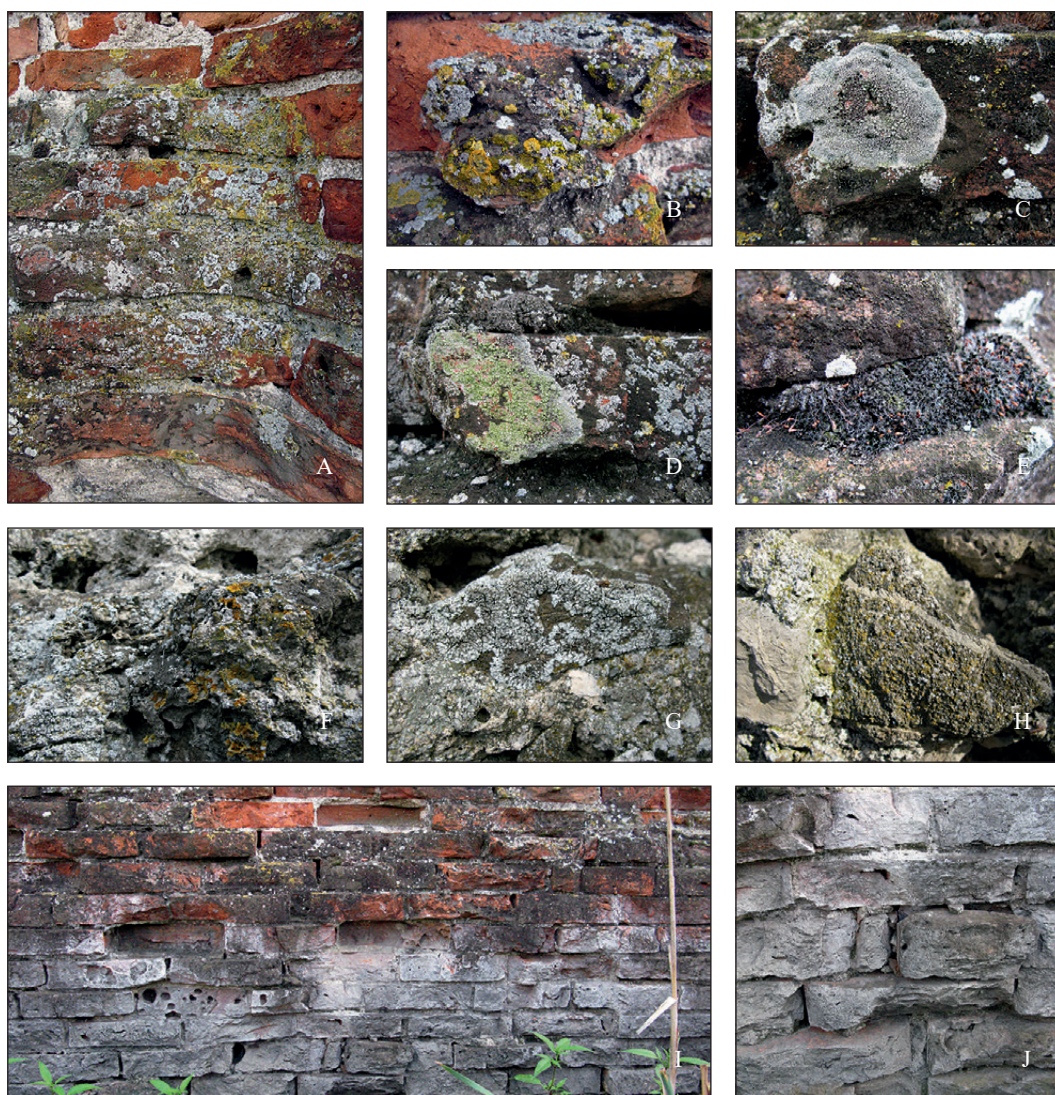
Fig. 6. Lichen and moss infestation of brick (A–D), mortar (E), and stone (F–H) of the pillar in September, 2022; lower, usually submerged part is discoloured and infestation free (I–J) (Archive of the PROTECTA project)
