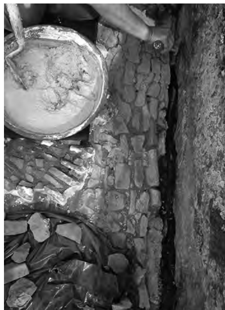
Fig. 3.2.15 : South-eastern part, when applying mortar in the space between the south wall and the tile floor (G. Çimen).
